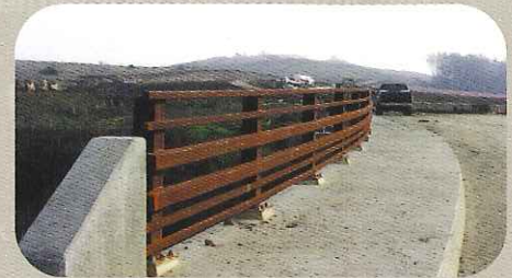
RADIUSED WEATHERING STEEL RAILING.
