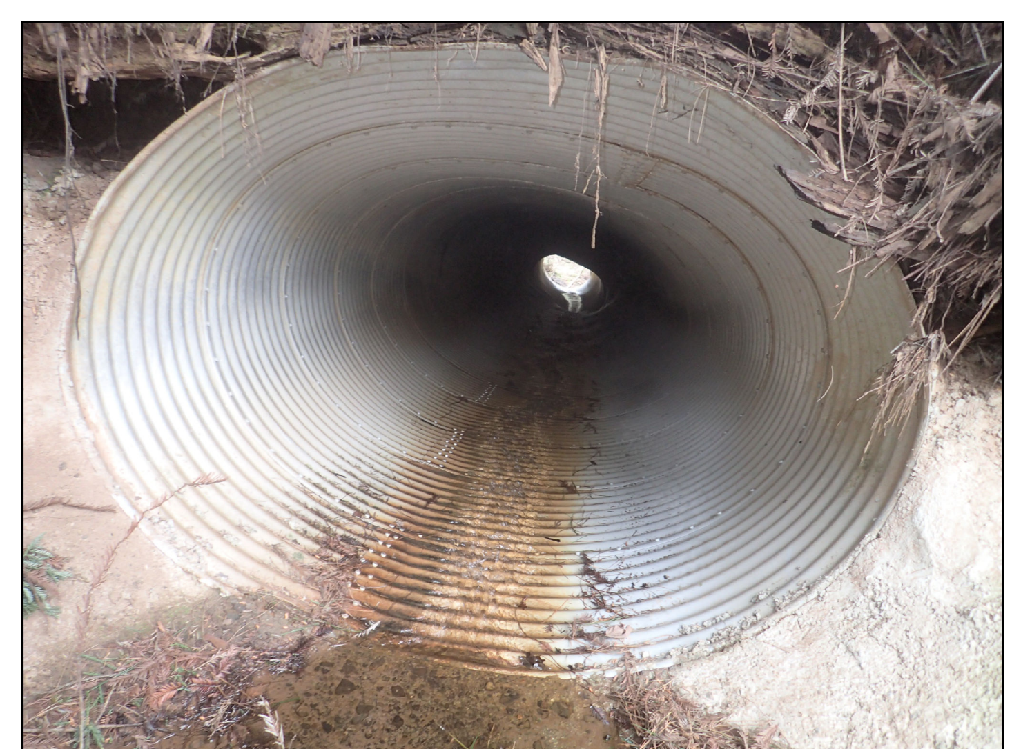
Photo 2. View of the culvert inlet. Note the deformation of the culvert and concrete used to repair the inboard fill face.
